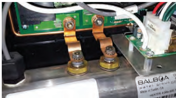
Close-up of the two copper straps that connect the heater to the spa pack circuit board.
